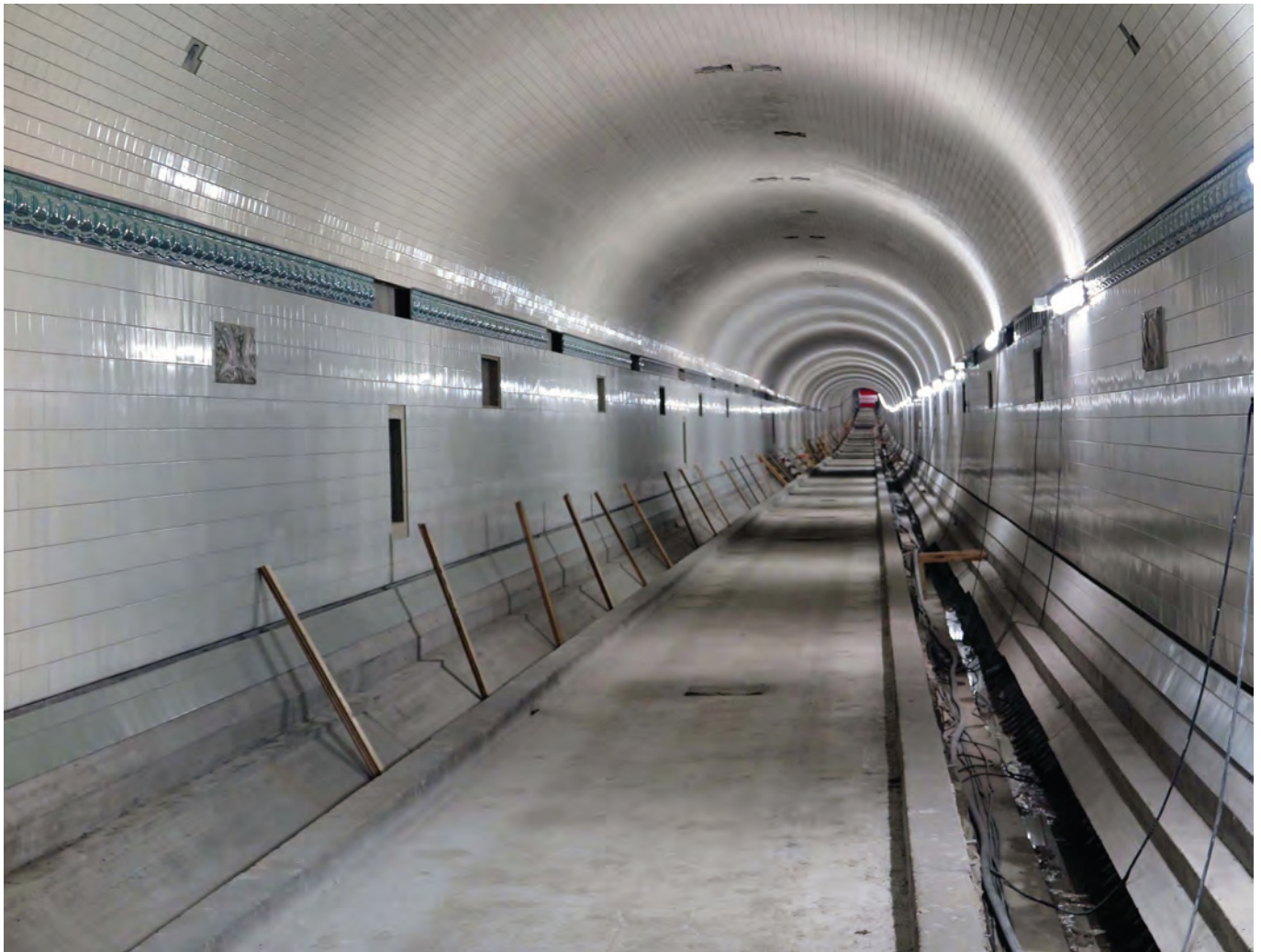
The easterly of the two bores of the Old Elbe Tunnel. This is nearing the end of a long restoration and we were fortunate to be granted permission to visit the works. The effort that has been taken to remove, restore and replace the original tiling is particularly impressive
